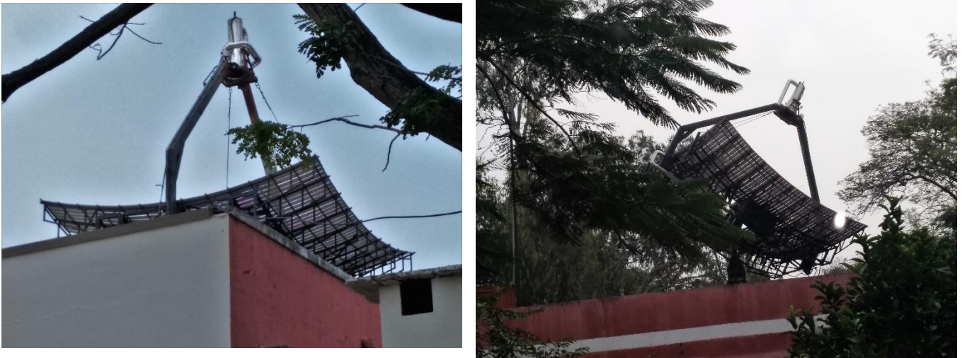
Fig. 6. CSP* Concentrated Solar thermal for power generation (ABD,TNAU,CBE-Dual axis tracking installation) ( ABD-TNAU coimbatore : Dual axis tracking of sun's movement)
