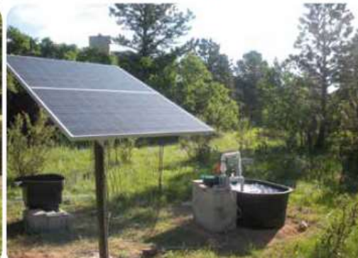
Images 18 & 19: Examples of surface and submersible water pumps
